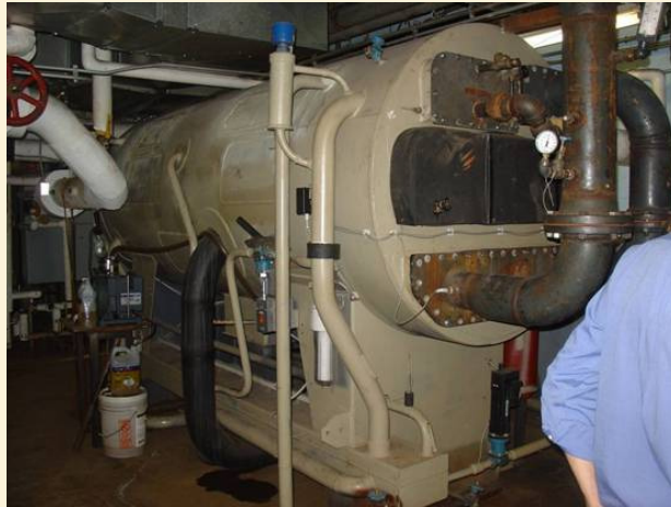
Long lifetime of absorption chillers. This one is > 70 years old !
